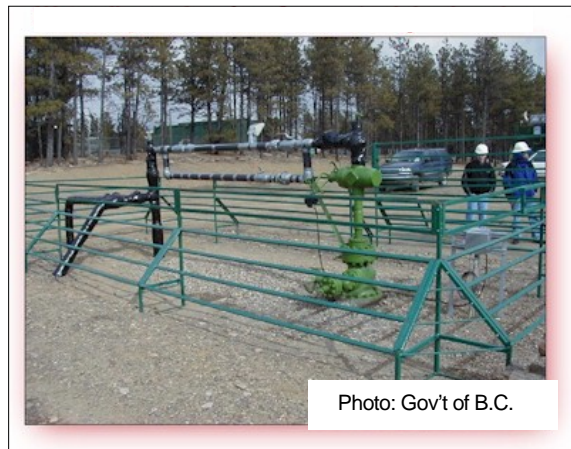
Water disposal for coal-bed methane development: subsurface injection site
